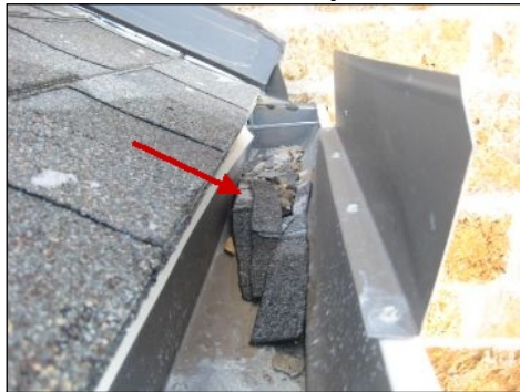
Construction debris in front elevation gutters
