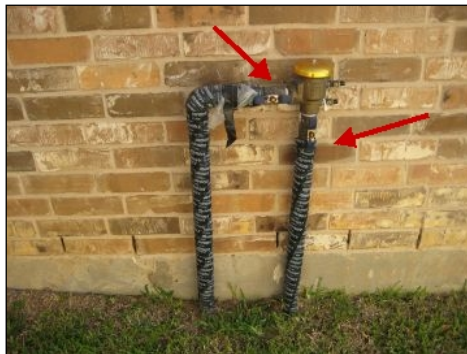
Main irrigation shut off valves on left elevation of home
