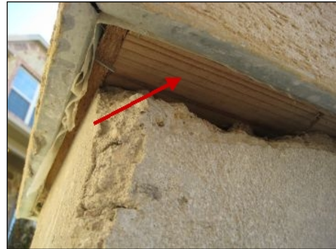
Exposed lumber at carport right column
