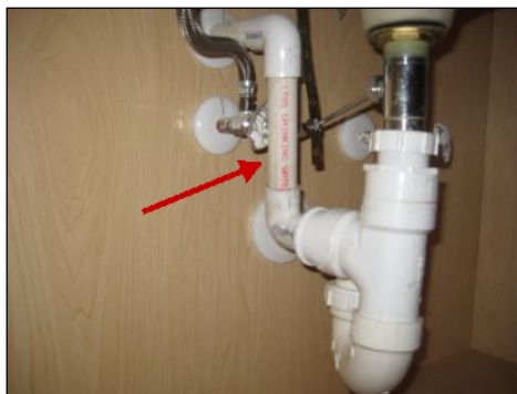
Primary A/C drain line at secondary bathroom
