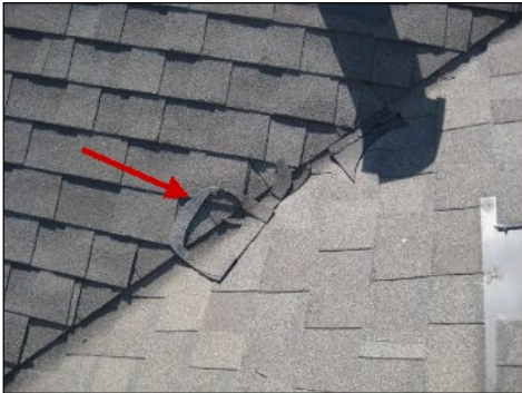
Debris on roof covering
