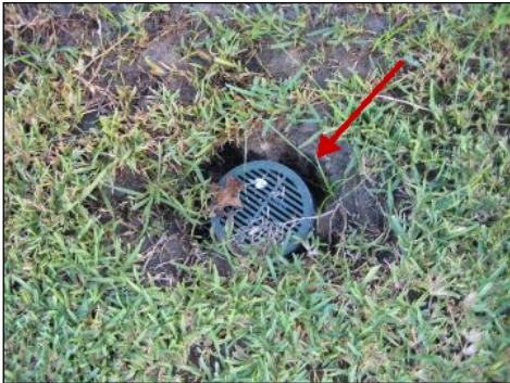
Grading void at drain on rear right elevation
