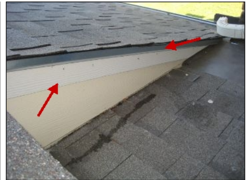
Siding and flashing missing sealant/paint at rear elevation
