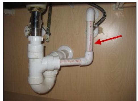
Primary A/C drain line at secondary bathroom
