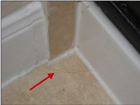
Cracked tile at front right bathroom
