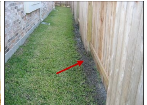
Moist area on left rear elevation fence line
