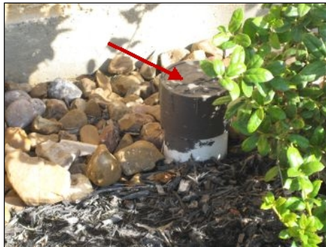
Main sewer clean out at front flower bed
