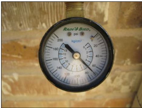
Water PSI at front left hose bib
