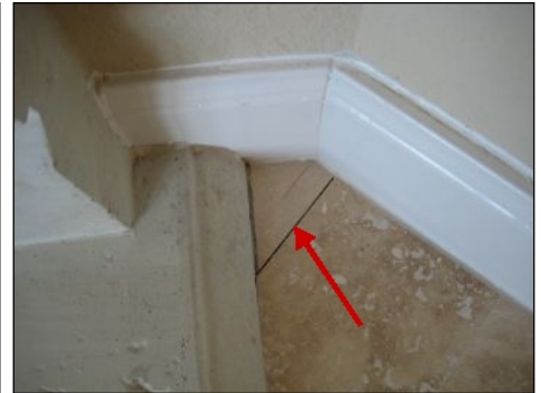
Crack in tile near fireplace
