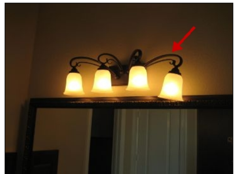
Master bathroom light not secure
