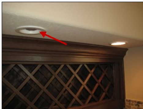
Light inop at wine bar in kitchen
