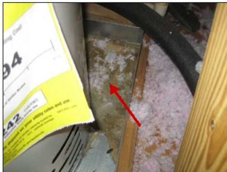
Debris in water heater drain pan
