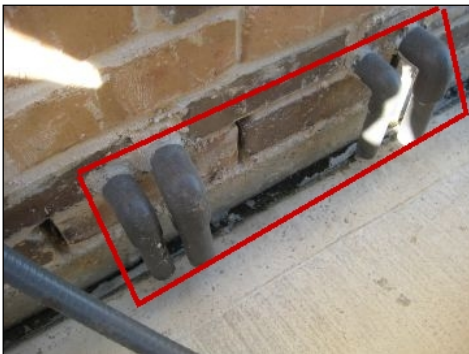
Water heater drain pipes at rear right elevation
