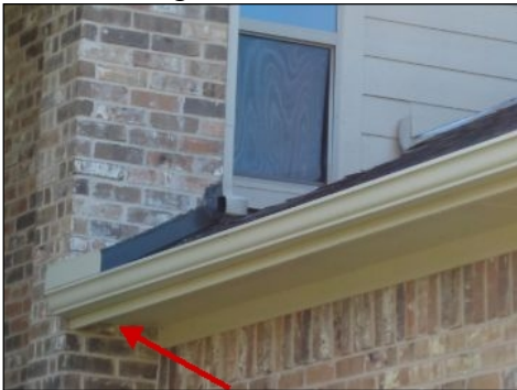
Recommend gutter down tube at rear elevation
