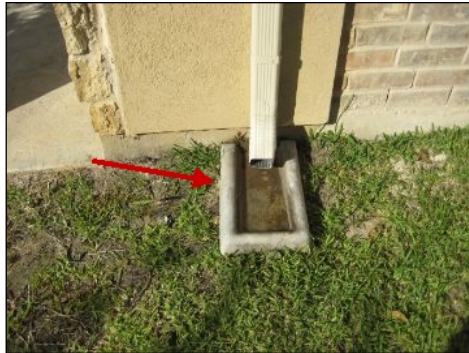
Splash blocks installed incorrectly
