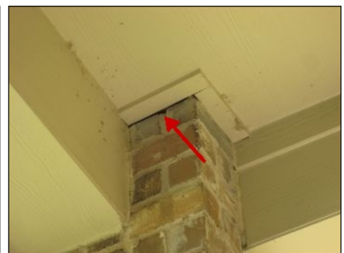
Seal gap at rear patio cover ceiling
