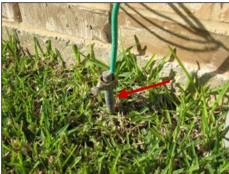
Lower ground rod at rear right elevation
