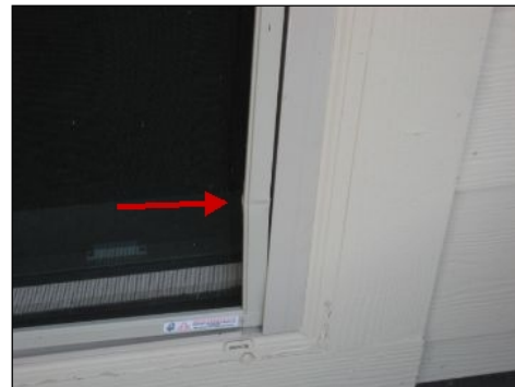
Damaged screen at second floor rear elevation
