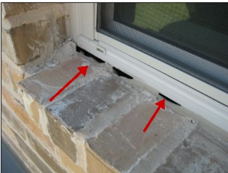
Gap at second story left elevation window
