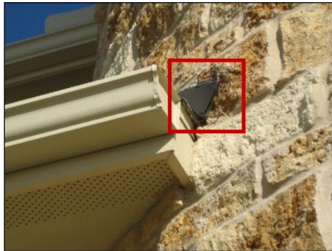
Missing kick out flashing at front elevation
