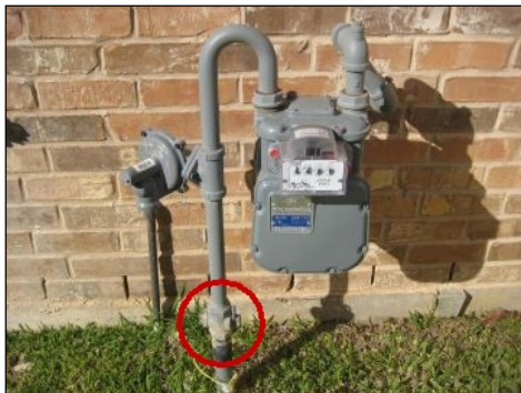
Gas meter and shut off valve on right elevation
