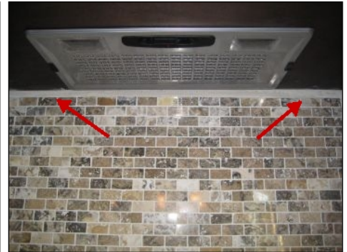
Tile backsplash not complete under vent hood in kitchen
