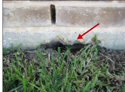
Void in foundation at rear elevation of home under master bedroom window
