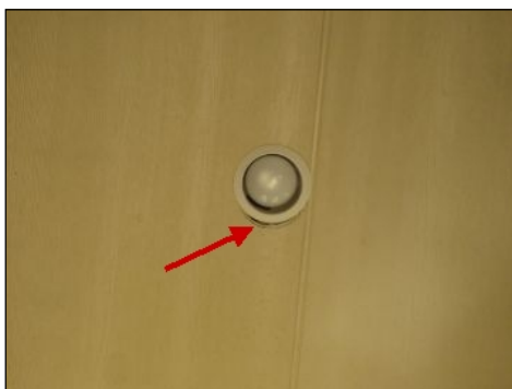
Gap at recess can light of front porch
