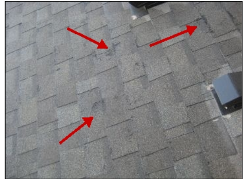
Deteriorated shingles at left elevation of home
