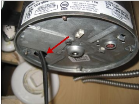
Disposer missing protective clamp
