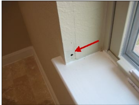
Drywall repair needed in utility room
