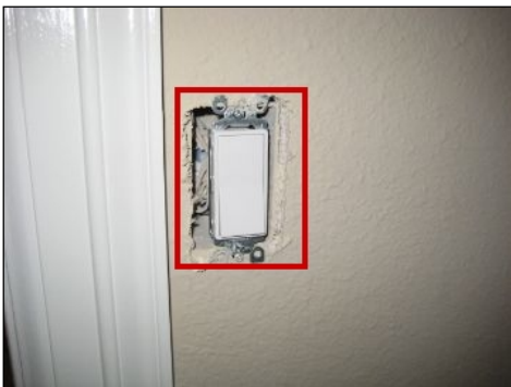
Missing light switch cover in coat closet
