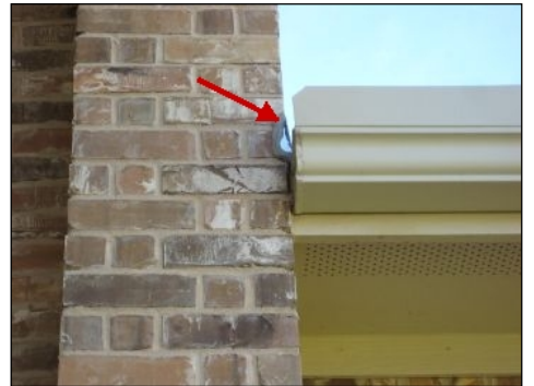
Missing kickout flashing at rear elevation near patio
