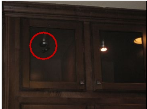
Light above fridge in cabinet inoperative
