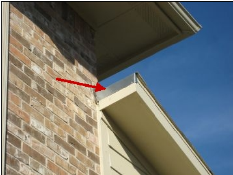
Flashing not painted at rear right elevation of home
