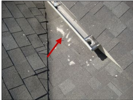
Paint/debris at front elevation
