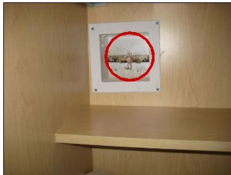
Gas shut off for cooktop in cabinet to the right of the unit
