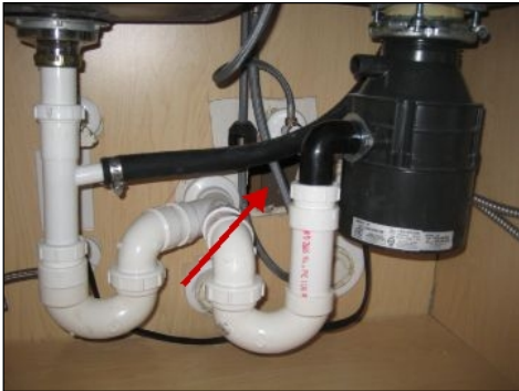
Seal gap under kitchen sink
