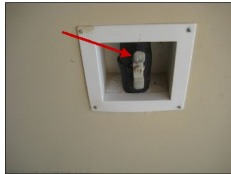
Main water shut off valve in garage
