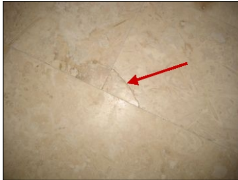
Cracked tile at living room floor
