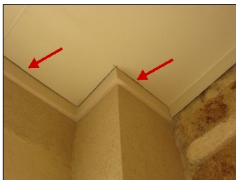
Seal gap at garage carport ceiling
