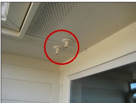
Secondary A/C drain lines at rear elevation
