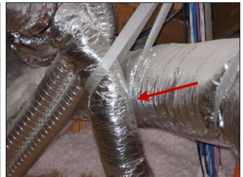
HVAC ducts in contact with one another
