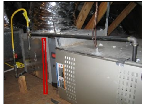
Support gas line to furnace in attic
