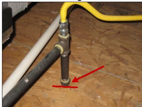
Unable to remove sediment trap cap at furnace
