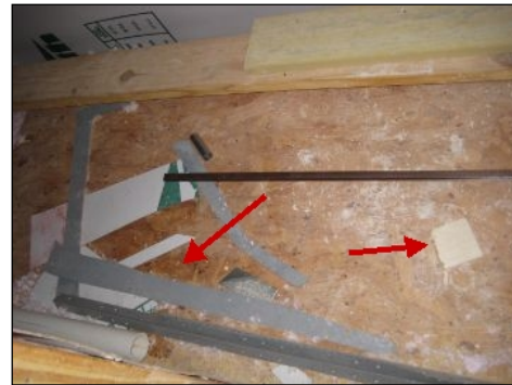
Debris in rear elevation walk in attic space
