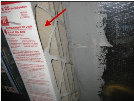
Recommend replacing HVAC filters at plenum
