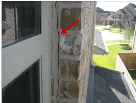
Crack in wall at second floor left elevation
