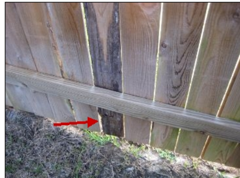
Fence picket deteriorated at front left side
